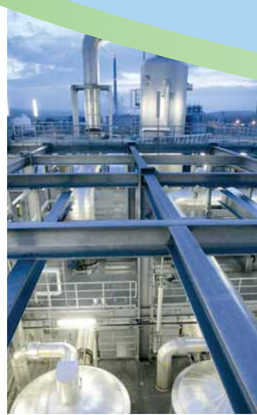
Bioethanol plant (Source: CropEnergies)
